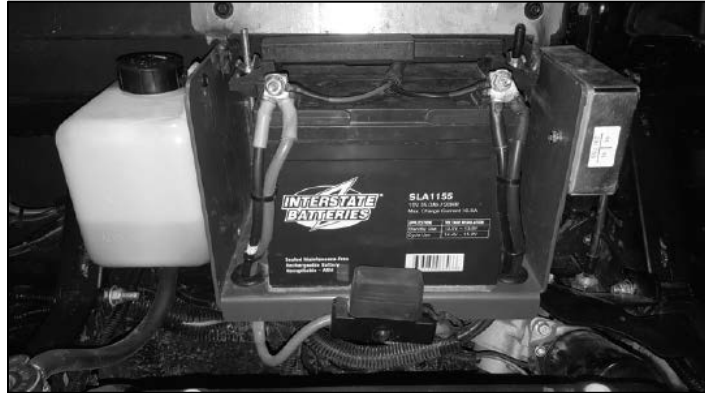
Figure 27: Battery Location Under Hood
